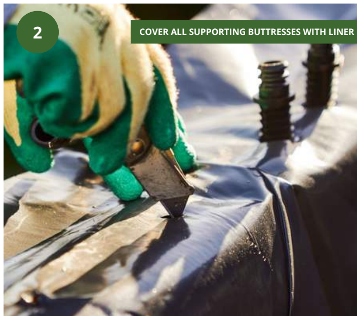
2 Get your liner into position - make small incisions for the final layer dowels to push through the liner.
