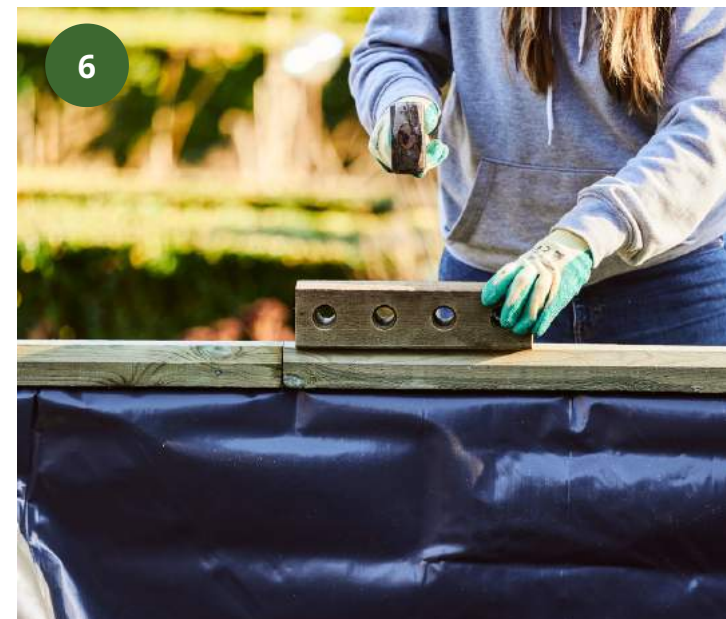
6 Knock on your capping layer - use a spare BlocX to protect the wood when hammering. JOB DONE!
