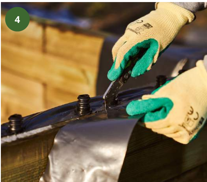
4 Trim excess liner with a sharp knife - using a retractable blade carefully cut away overhanging liner.
